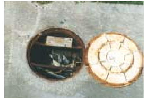
Tank Basin Automated Leak Detection/Gauging Equipment
